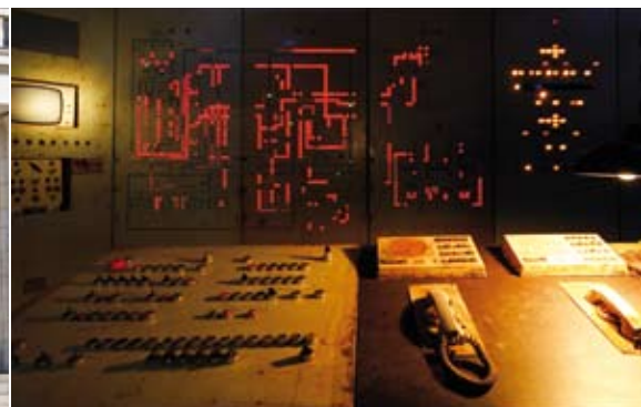
Technology in the Eichenthal Bunker
